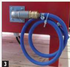
3 Inert gas entry
